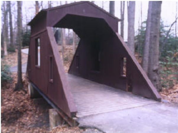
LAKE ANNE, 22', 1984, pedestrian, 46-29-B. Across a brook in Reston, Fairfax County, VA. Wiehle Av. (SR828) S. 0.25 miles from jct with SR606 in Reston, W. on North Shore Dr. 0.15 miles (1 block), S. on Northgate Sq. to the bridge on the E. side of the road. May, 2003. Photo by Don Burnell.
